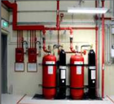
Automatic Fire Suppression System
